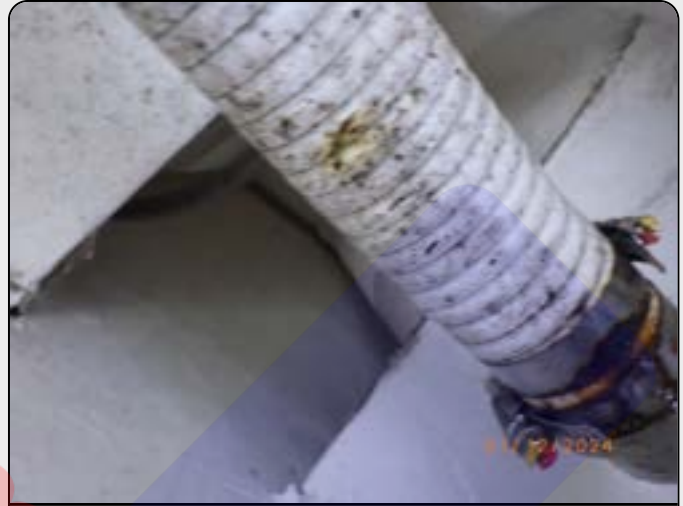
Photo 31: Leak coming from above
