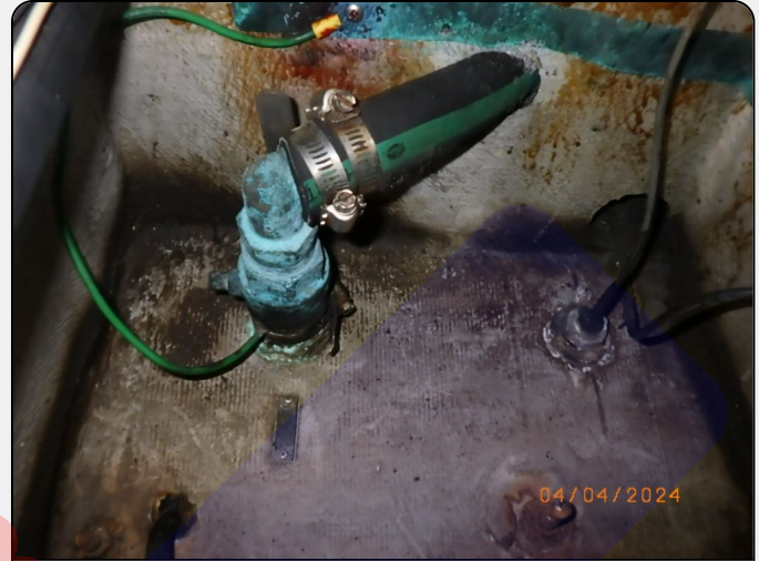
Photo 6: Engine room - no movement
